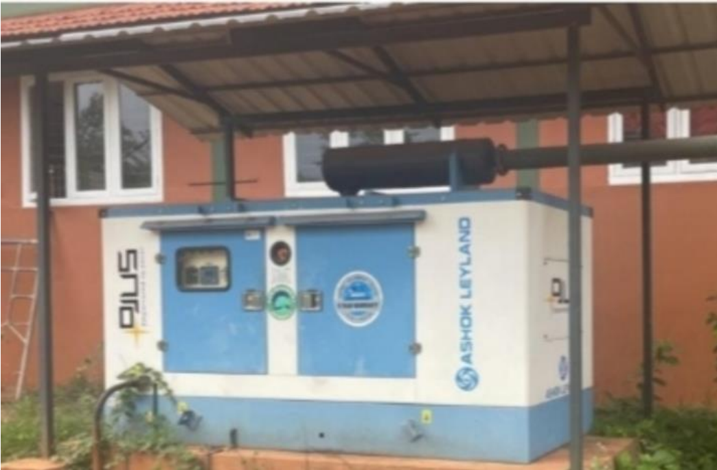
Figure 7: The silent Generator installed in the college
